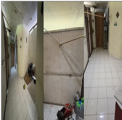
Figure 2. Musholla before renovation: Condition of the local musholla at Taman Mejuah-Juah prior to the community service intervention
